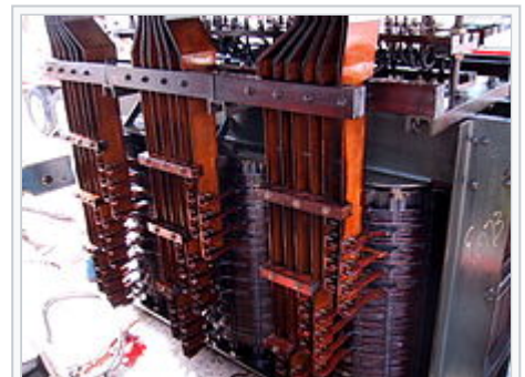
In an electric arc furnace , the transformer has a heavy copper bus for
