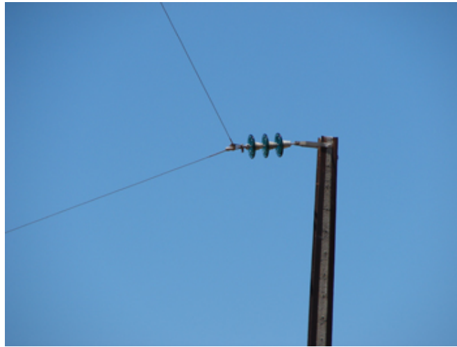
19kV Single-Wire Earth Return wire in Australia
